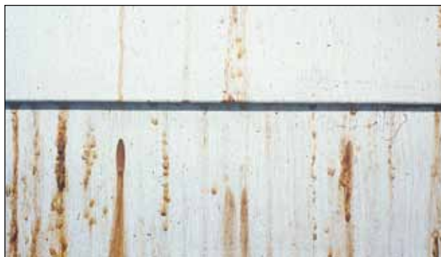
Figure 16–26. Water-soluble extractive discoloration can result from water wetting the back of the siding and then running down the front of the board.
