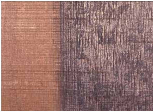
Figure 16–18. Front view of exterior grade of plywood siding after 10 years of exposure. The right-hand portion was exposed to the weather, whereas the left-hand side was covered with a board to give a board-and-batten appearance.
