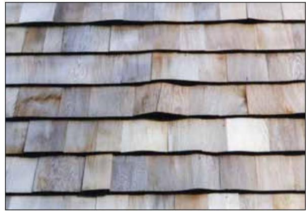
Figure 16–17. Shingles installed with insufficient gap later warped when they expanded after getting wet.
